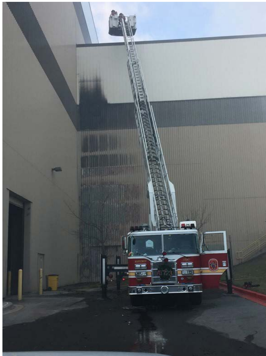
Figure 12 Blistering paint on the tipping floor south wall (12/08/2016)
